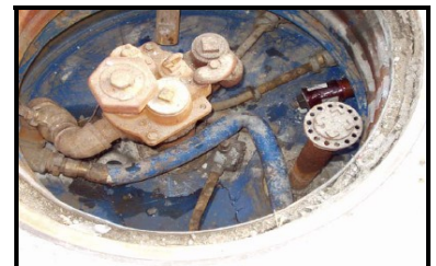
Flexible piping is kinked
