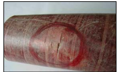
Fiberglass piping is cracked
