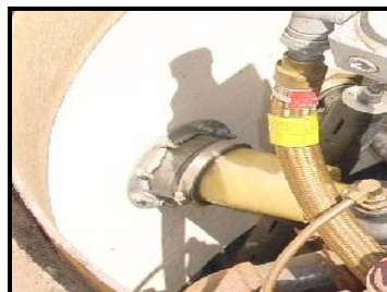
Sump penetration seals in good condition
