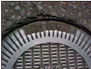
Cracked spill bucket lid
