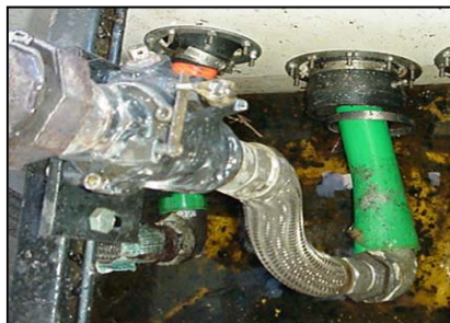
Metal flexible connector is twisted due to growth of flexible plastic piping
